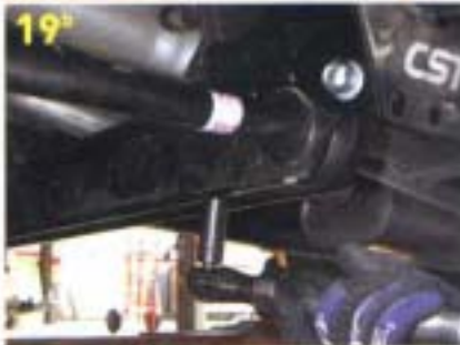
19 WITH A SPECIAL TOOL, THE KEYS ARE CRANKED UP SO THE KEEPER PLATES CAN BE SLID IN THE HOLE. ONE IN THE BOLTS IS RUN UP LOADING THE TORSION BAR.
